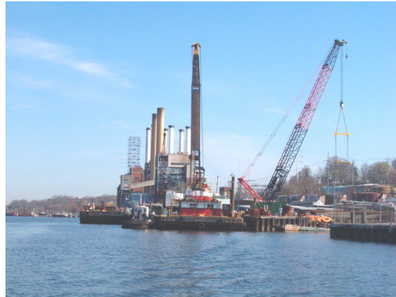
Cranes and barges at former Hinfin property—staging area for Roslyn Viaduct construction.
