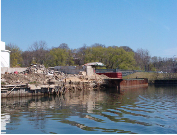
Collapsed bulkhead on north side of Glen Cove Creek.
